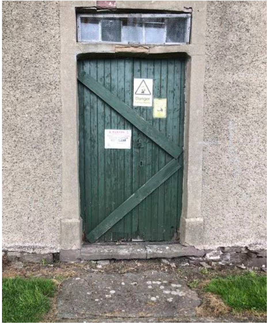
GD02 and TW01 - South doorway in the base of the tower © Andrew Rodger 2021
