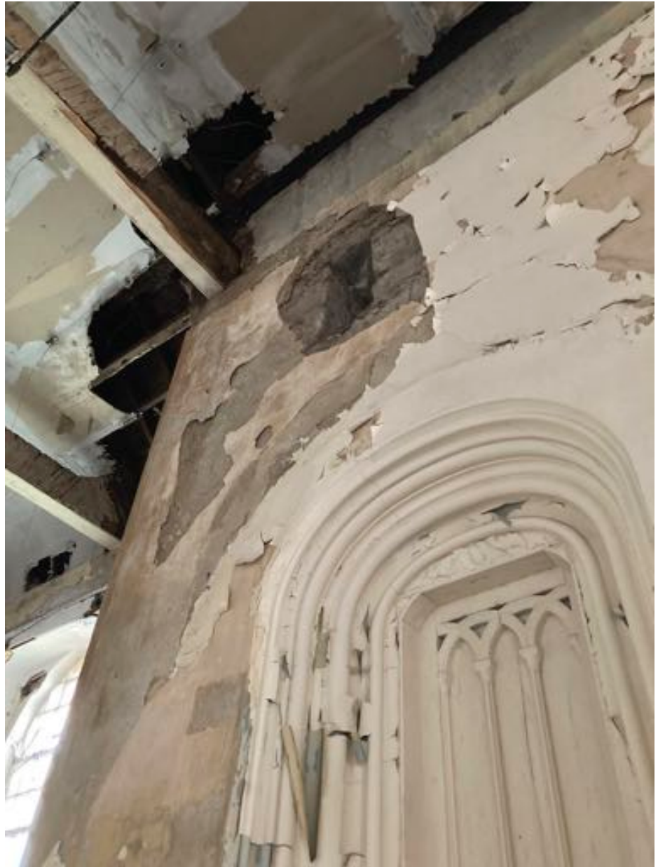
North wall of the tower in the main volume. It shows the recessed doorway from the tower into the now absent pulpit. It also shows the shot hole above but there is no obvious evidence of the timber canopy, as described by Macara. © A. P. Rodger 2021
