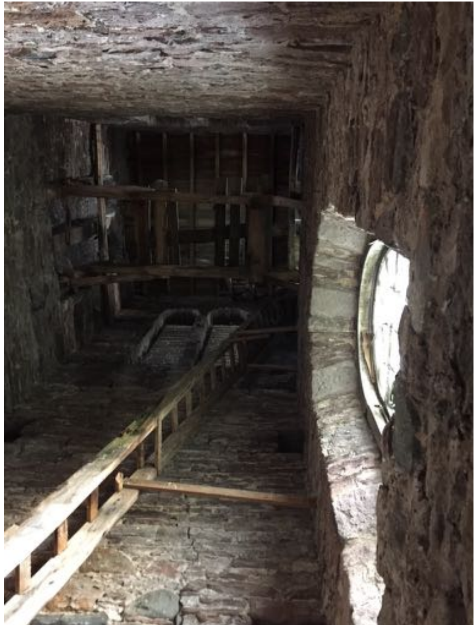
View of the tower from the mezzanine level © Andrew Rodger 2021. Note the running crack on the east wall which is replicated to a lesser degree on the west wall and which aligns, more or less, with the intersection with the main south wall outside face but also relates to the blind window cavities in the wall thickness.
