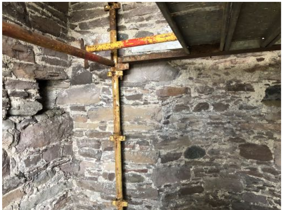
Level 3 view of north west corner of tower, showing typical putlog and the top of the curved recess in the north wall © A. P. Rodger 2021
