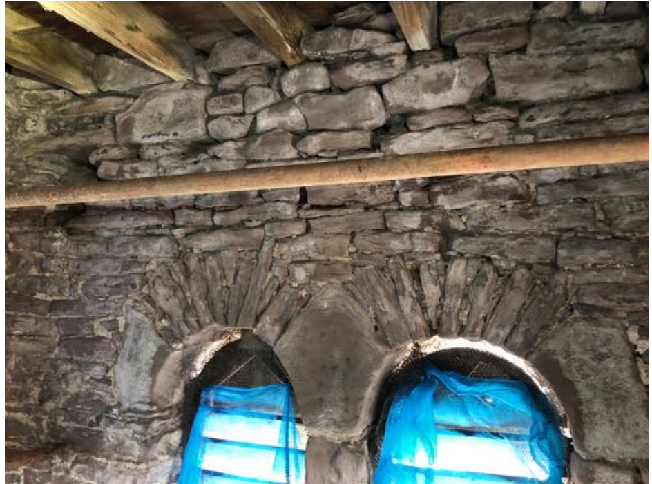
West wall of level 4 showing the unstable roof joist bearings © A. P. Rodger 2021
