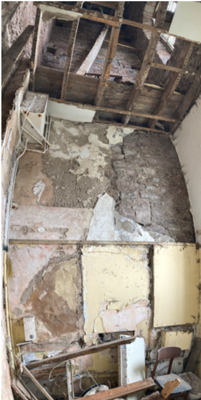
Tower view from the entrance to the mezzanine level showing Tier 3 and part of Tier 4. Note the crack, referred to in the text, which is mirrored, to an extent, on the opposite wall of the tower.tower
