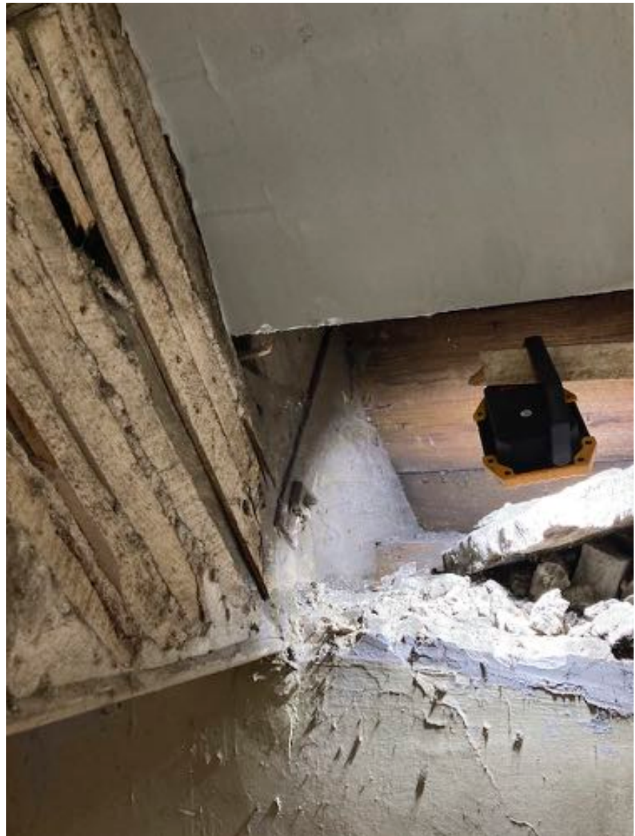
A typical truss bearing, this being the south end of the truss nearest the dividing wall above the main hall. In it you can see the lathing to accept a plaster coating and the edge bead of the timber applied to the underside of the beam. Also an iron bracket holding the rafter foot onto the beam. Note the plasterboard applied as part of a whole ceiling repair. © A. P. Rodger 2021
