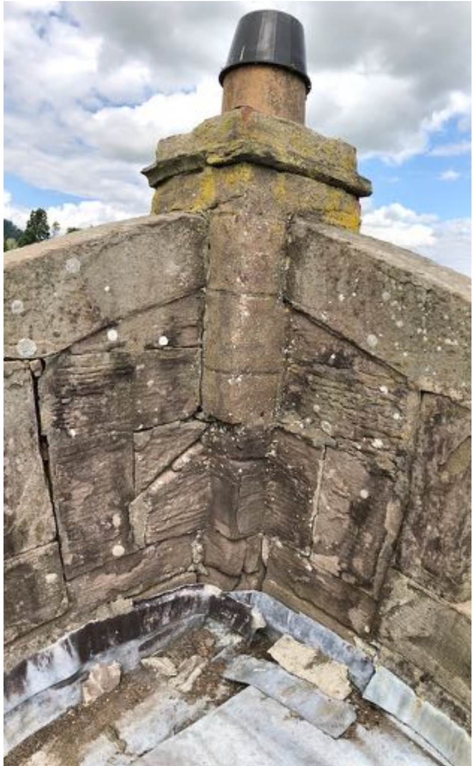
View of the north east corner of the parapet showing the rebuilt section. The only stone which bonding across the parapet is the broken one with its bed approx. 120mm above the raggle. Above this stone the pier is formed with unbonded brickwork. © A. P. Rodger 2021
